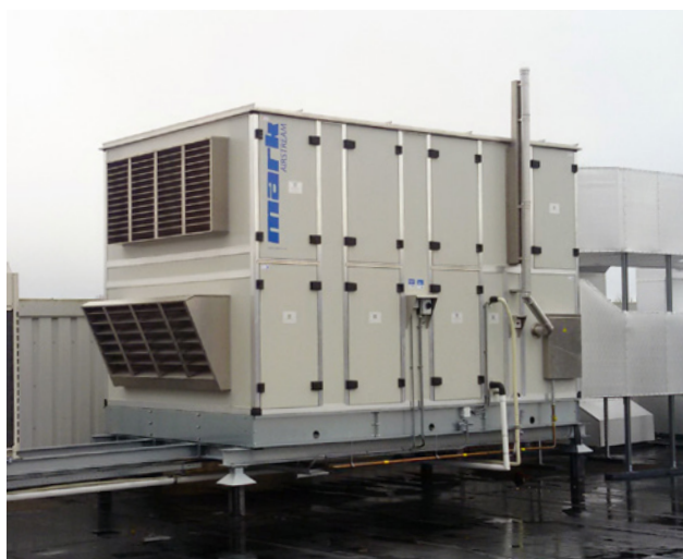
AIRSTREAM wtw-unit in buitenopstelling.
