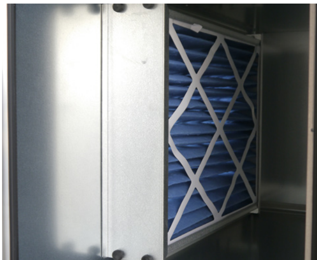
Filter in de unit.
