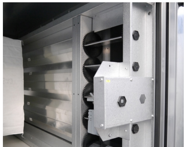
Bypass in de unit.
