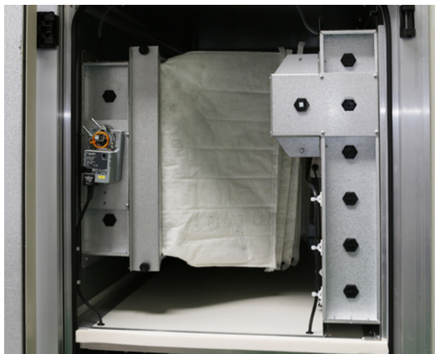
Filter in de unit.
